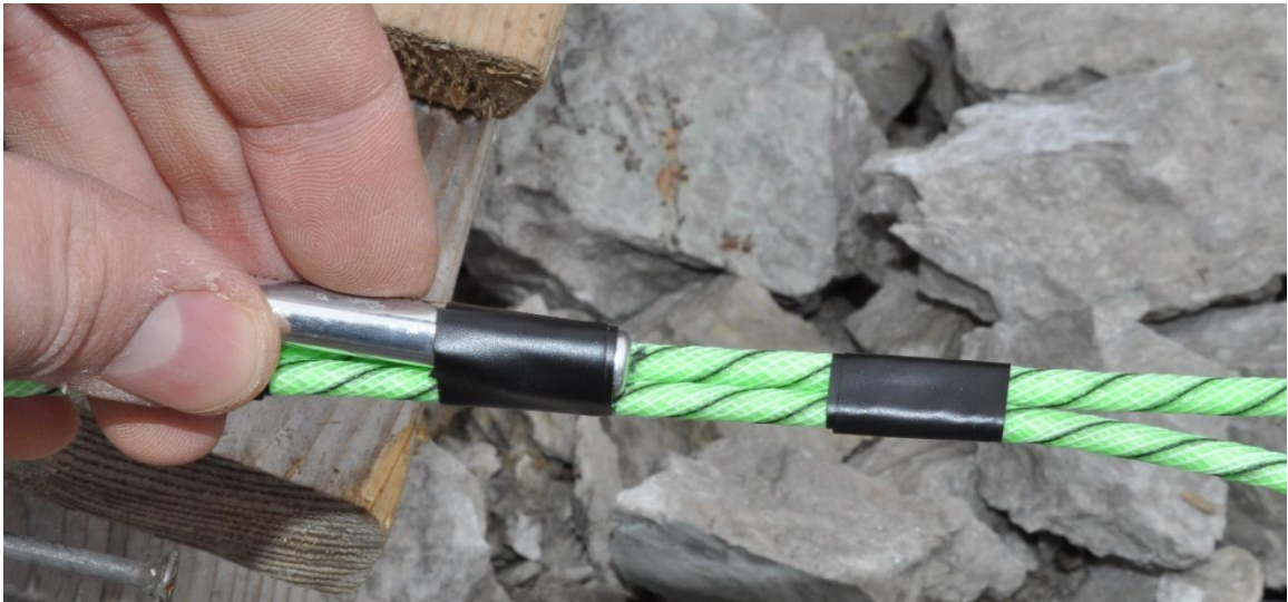
Figure A. 8: Securely attach the blasting cap so that it is in line with the measured marks
